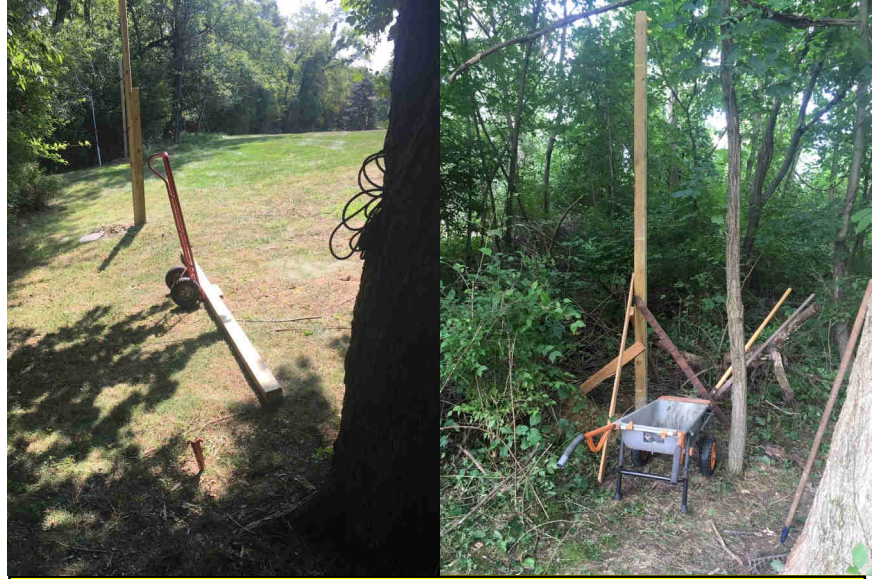
Antenna construction has begun! Photos courtesy of and © Copyright 2019 William R. Hill W3WH
