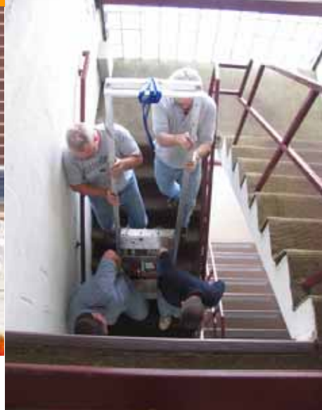
Walking the repeater rack down the steps from the roof to the elevators
