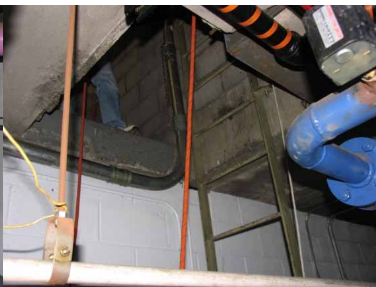
How you access the comm equipment from the mechanical room
